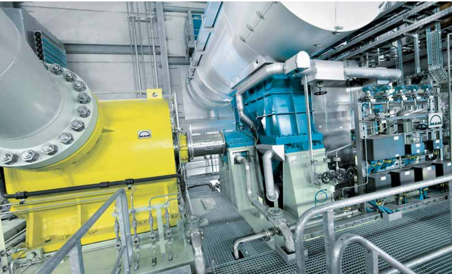
RV080 pipeline compressor and DK 63/130 steam turbine. Output: 22 MW
